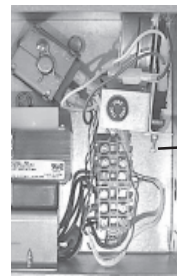
Figure 37B - Junction Box with AquaSaver® Controls
