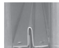
Figure 46C - The end of the top connector on the "open side" of the connector assembly.
