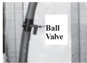
Figure 36 - Disconnect the power and use ball valve to adjust water flow
